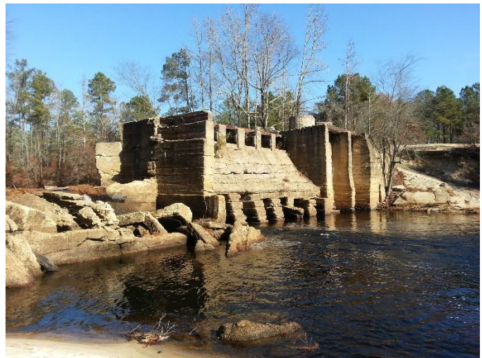
View of breached Unnamed Dam A taken on site visit, November 2012 with Fort Bragg, Dial Cordy and Associates and American Rivers.
