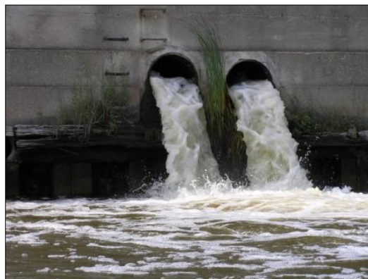
Combined sewer overflow in Chicago
