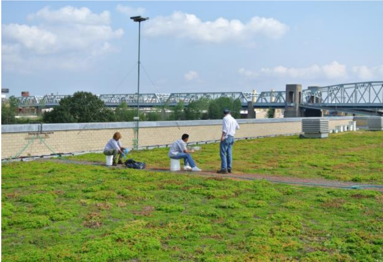
Maintenance work being undertaken at the New York Parks City-wide Greenroof Project.
