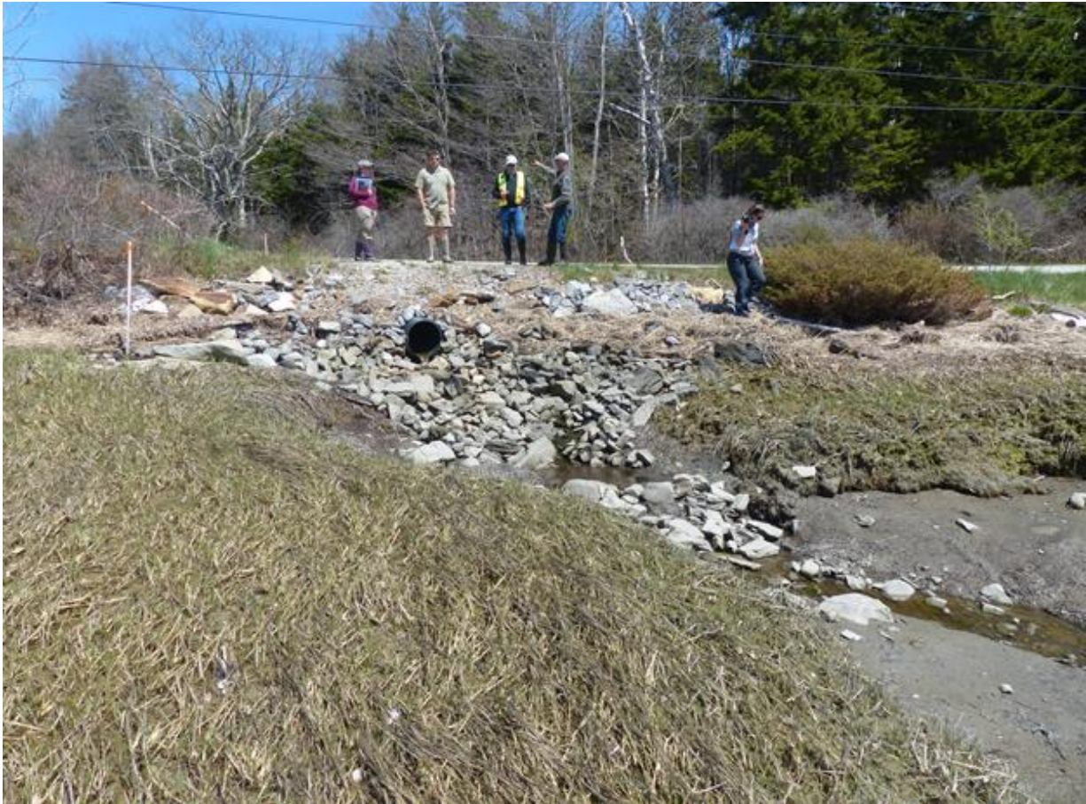
Figure CS3-1. This small culvert under Basin Point Road sits about four feet above the tidal flat surface. During extreme tides, water has been observed as high as the edge of the pavement.
