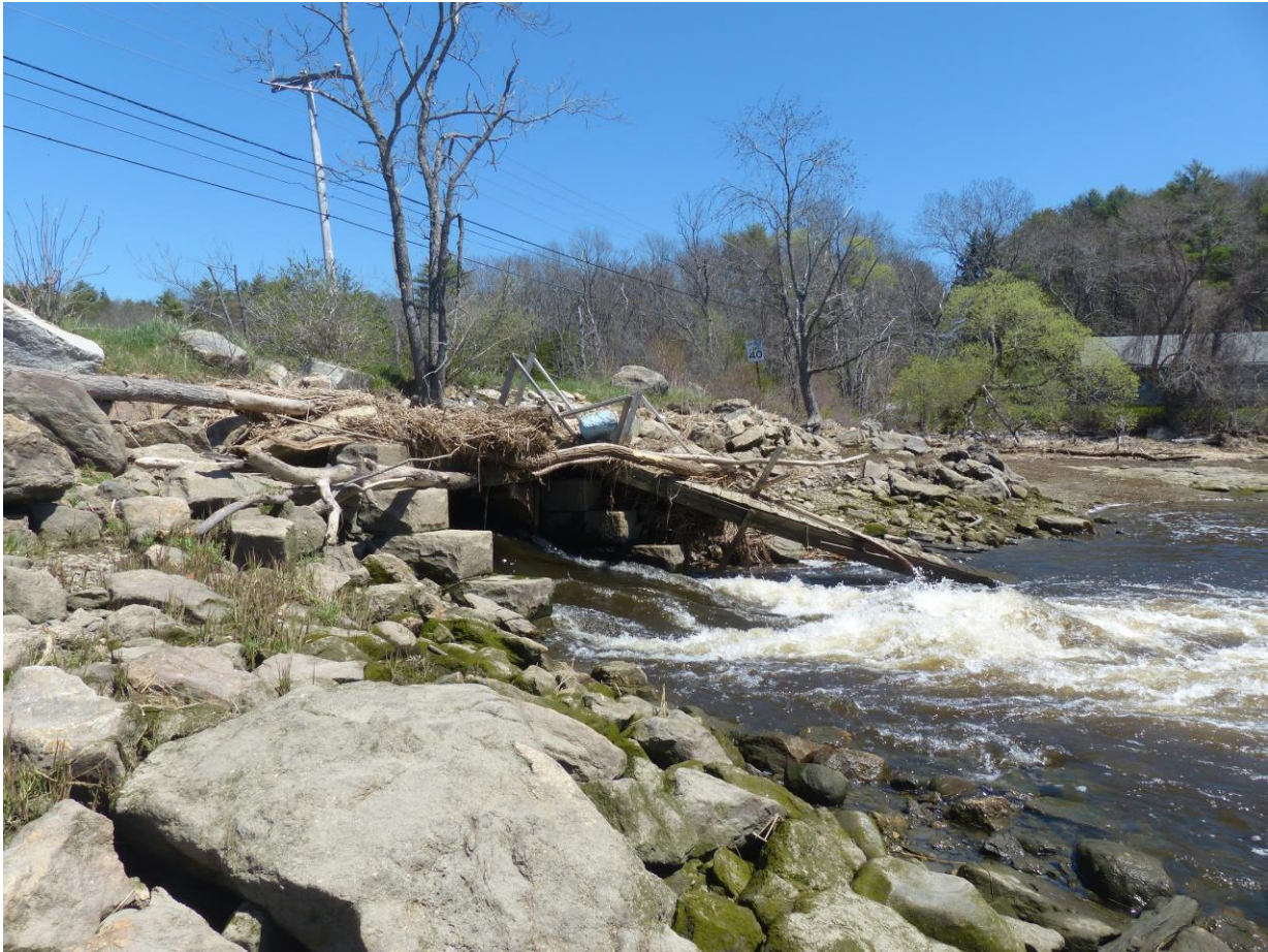
Figure CS2-1. Downstream view of the under-sized culvert under George Wright Road. Built in the 1930s, the culvert is completely submerged at high tides. Photo shows water forcefully exiting the culvert as tide recedes.
