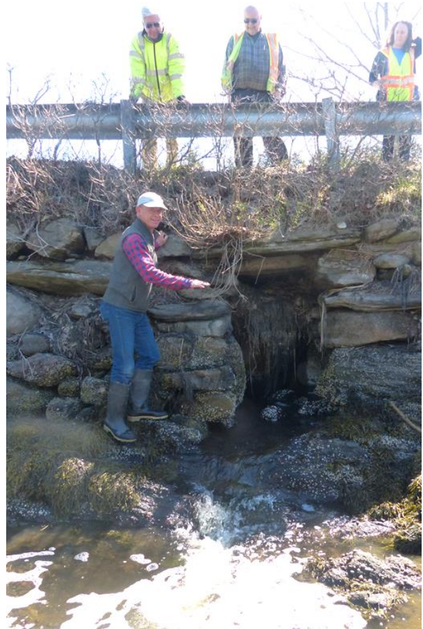
Figure CS1-1. Stone structure under Route 216. Structure has logs at the top level supporting the stone under the roadbed and what appears to be a collapsed rock in the center that only leaves a small gap for water to flow. It severely limits tidal flow to over 13 acres of wetland upstream.
