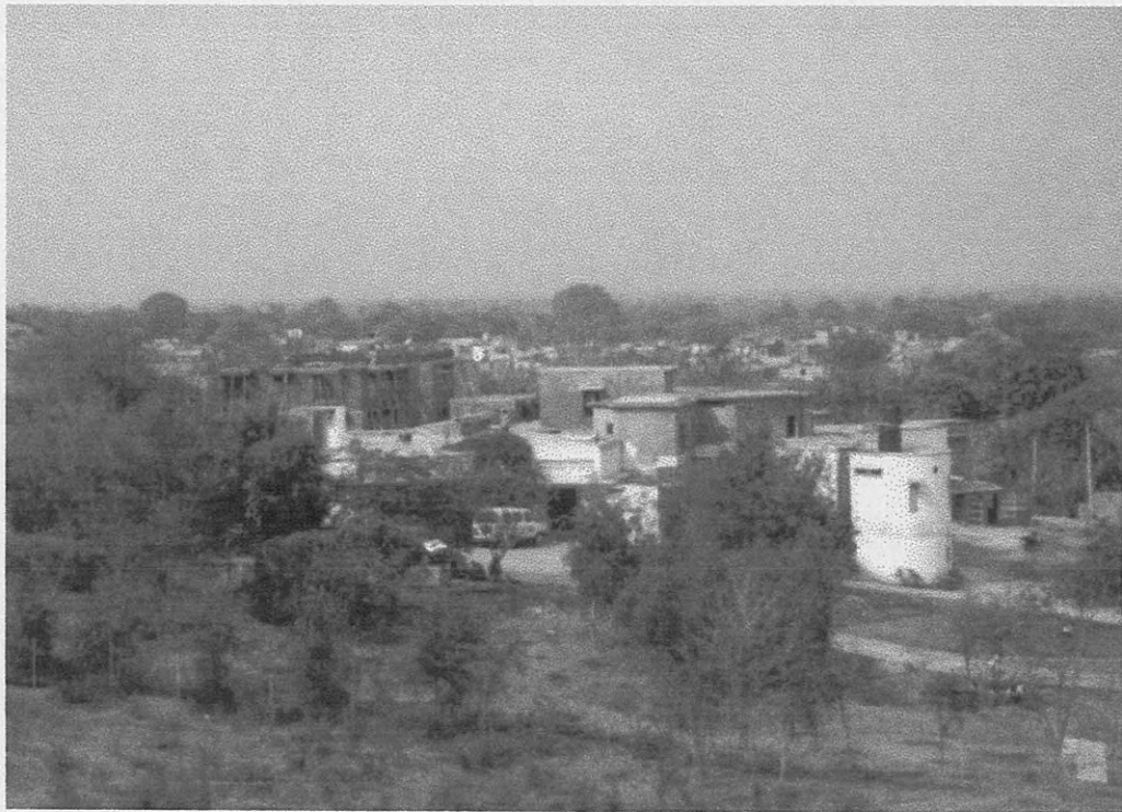
CONSTRUCTION OF THE NEW DOCTOR'S AND NURSES RESIDENCE SUPPORTED BY THE DAVID SHEPHERD CONSERVATION FOUNDATION, U.K. AND ESSO INDIA PVT. LTD .
